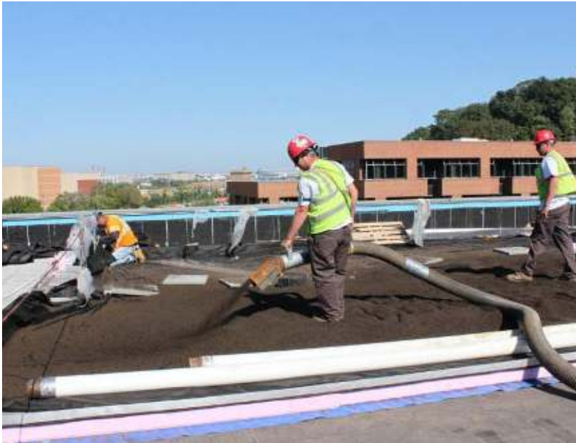
Media was pneumatically conveyed and blown on the roof in the 1 st phase.
